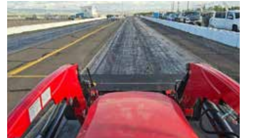
The track view from the tractor that helps put down new rubber.
